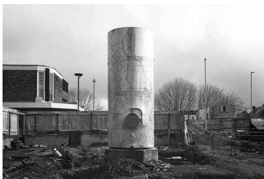
Infrared photograph of a heat storage tower during construction, Hebburn, Paul Dolan, 2023
