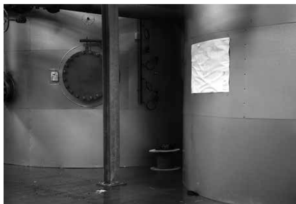
Heat storage tanks, Jarrow, infrared photograph, Paul Dolan, 2023
